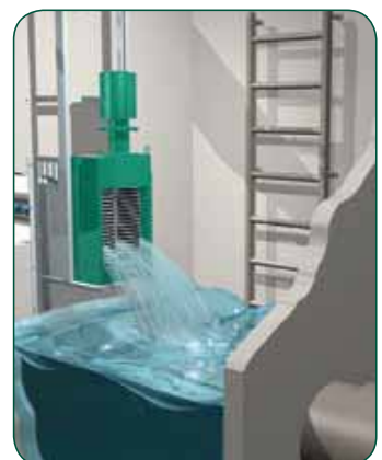
Muffin Monster in Pumpstation
