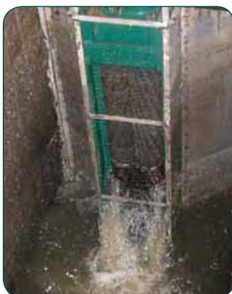
Muffin Monster in Pumpstation
